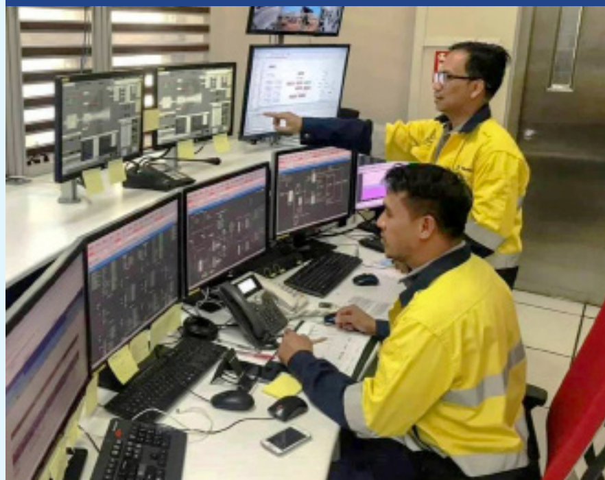
Operations personnel at work in Avion power plant
